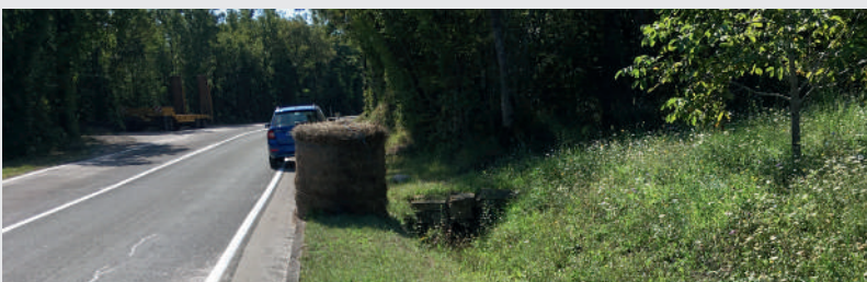
Concrete drain not protected
